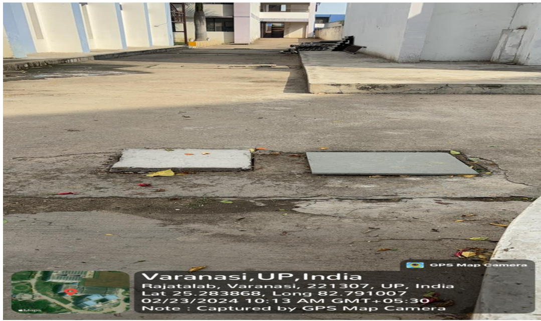
Figure 11: Drainage for collecting liquid wastes from various originating source.
