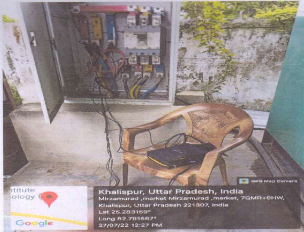
Fig-4.2: Checking Load & Electrical Parameters through Load Analyzer
