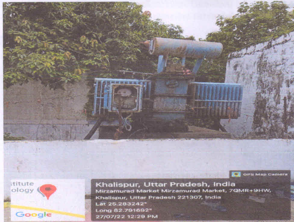
Fig-4.1: 11/0.4 Transformer (650 KVA)
